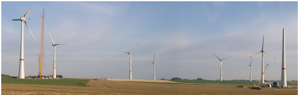
Fig. 5 First wind farm consisting of 7.5 megawatt (MW) Enercon E-126 turbines, Estinnes, Belgium, 20 July 2010, two months before completion.
