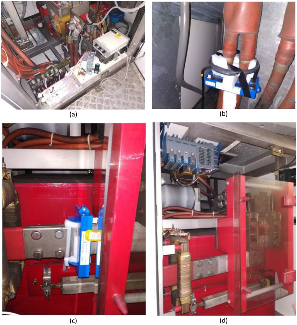
Fig. 6. Installation of the DAS and transducers: a) voltage transducer and supply systems for the active sensors and the DAS; b) Rogowski coil for the i_r measurement; c) HOP sensor for the i_p measurement; d) DAS.
