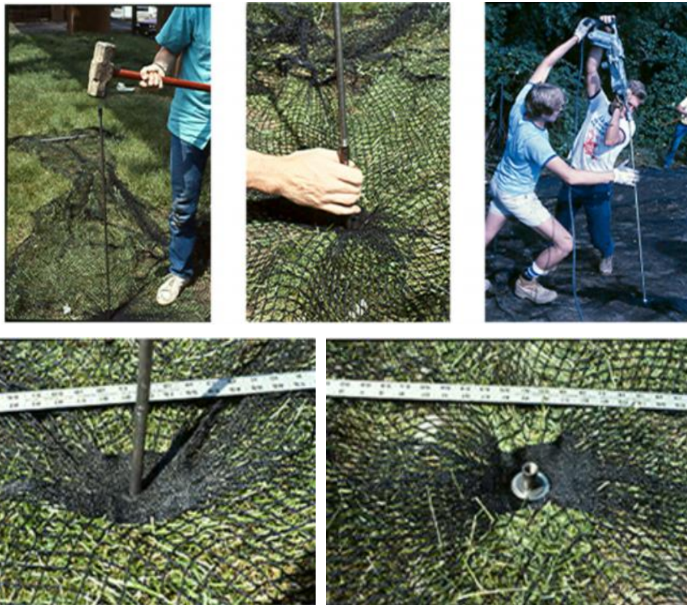
Fig. 2.30. Field deployment of anchored geosynthetic covering system using flip anchors on unstable silty clay slope (Koerner, 2015).
