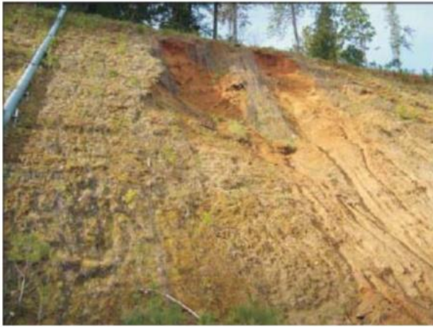
(a) Surficial slope failure
