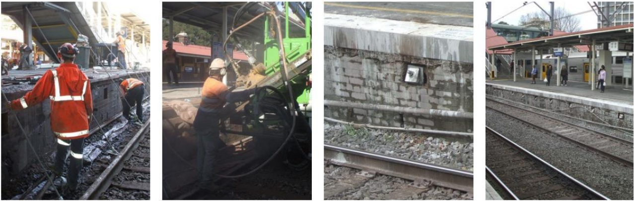
Fig. 2.35. Application of flip anchors (HULK anchors) to reinforce the platform six at Redfern Station NSW, Australia, (Anchoring Rope and Rigging Pty. Ltd., 2021).
