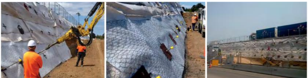
Fig. 2.37. Application of flip anchors (Platipus anchors) to support M4 Motorway, Sydney, Australia, (Platipus Anchors Limited, 2021).
