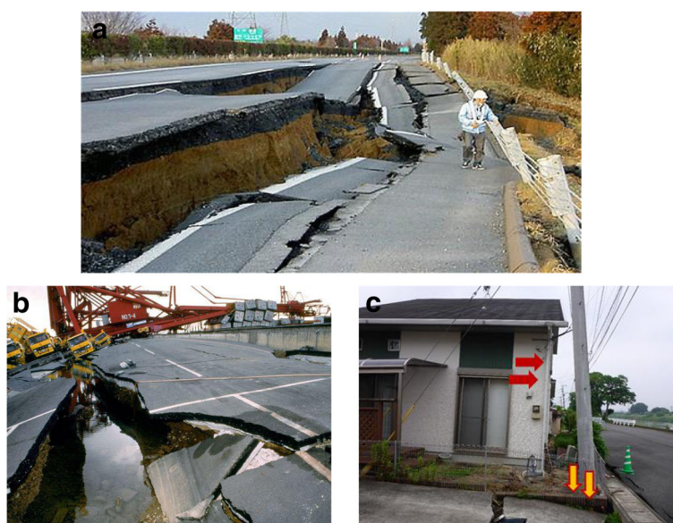
Fig. 1 a Damaged road due to liquefaction in the Great East Japan earthquake. b Damaged road due to liquefaction in the Great Hanshin earthquake, Japan. c Tilted house due to liquefaction in the 2016 Kumamoto earthquake, Japan
