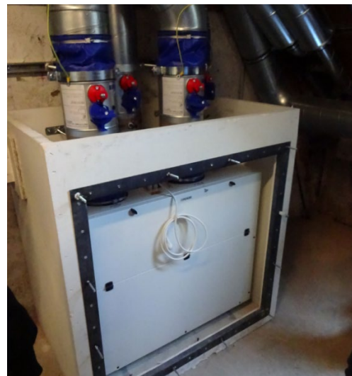
Figure 3-6 Central unit with fire protected housing and fire dampers at the top. The fire protected maintenance cover at the front is not mounted at the moment.
