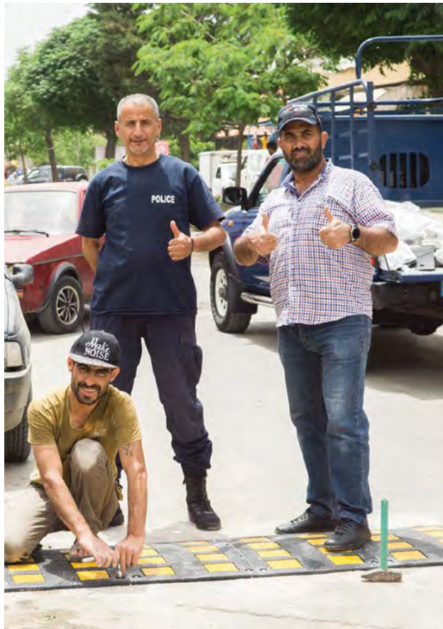
Bar Elias police together with a local worker & citizen scientist install the speed humps
