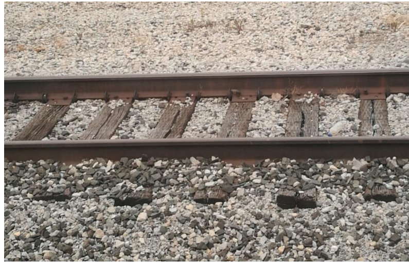
Figure 2.2 Ballasted railway track with rotten timber sleepers.
