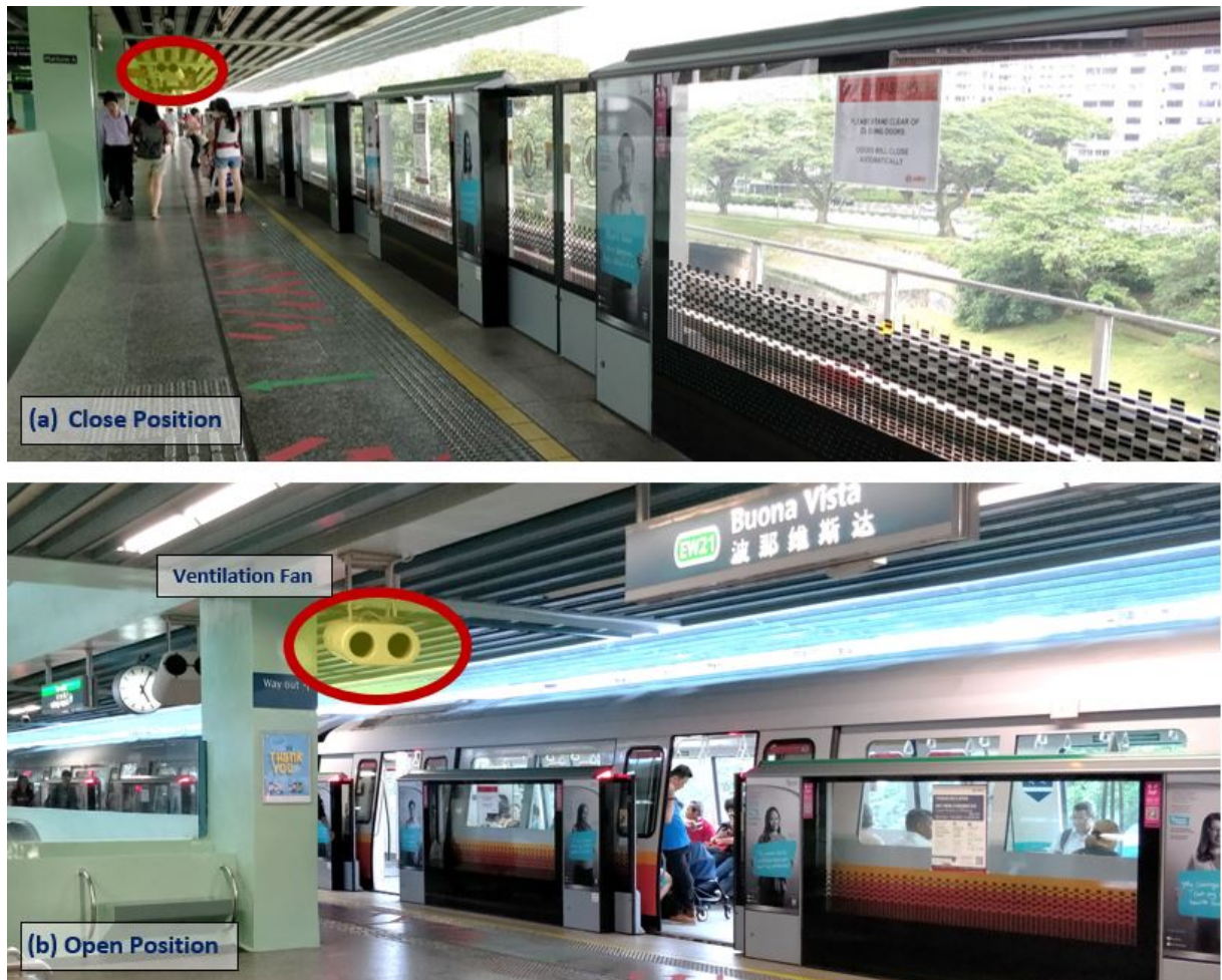
FIGURE C.2: Half-height PSDs in Above ground Stations of the East-West MRT Line, Singapore, Featuring Platform Ventilation Fans [a, b] (Author)
