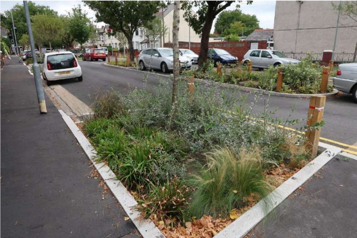
Fig. 14: The Greener Grangetown scheme was delivered to remove surface water from combined sewer networks, to avoid needing to pump effluent 8km to a sewage treatment
