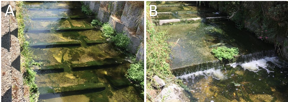
Figure 7.60. A bridge apron divides the upstream and downstream sub-sites along the Mangarau Stream. A: Baffles with alternately placed gaps span the length of the structure. B: A drop on the lower end of the bridge apron may act as a fish barrier.
