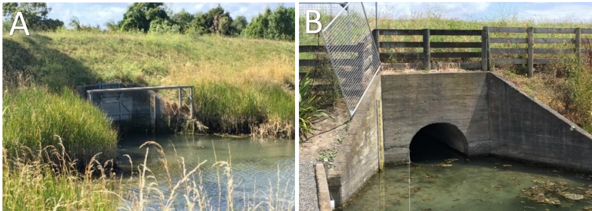
Figure 7.79. A flood gate and a pipe culvert divide the upstream and downstream sub-sites along Memorial Park Drain. A: The flood gate covers the width of the culvert's outlet. B: The culvert's inlet allows upstream water to drain into the downstream sub-site when the flood gate opens.
