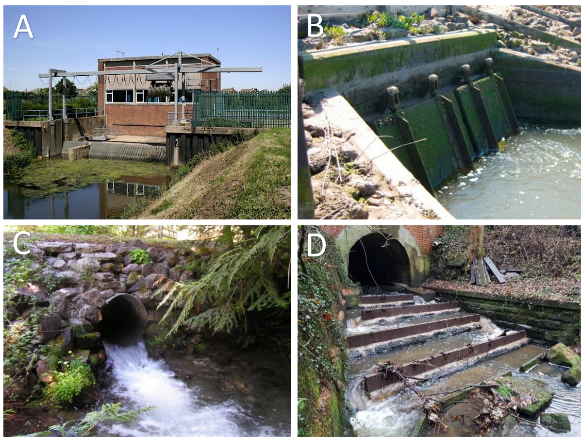
Figure 1.2. The drainage structures used in this study are expected to look similar to those above: A: Chain Bridge Pumping Station, Lincolnshire, UK (Black Sluice Internal Drainage Board, 2016). B: Flood gate along the River Stiffkey, Norfolk, UK (Wright et al. , 2016). C: Pipe Culvert along Clugston Creek, Washington, US (INVW, 2019). D: Bridge Apron along the Cong Burn, UK (Wild Trout Trust, 2018).
