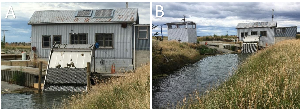
Figure 7.104. A: A pumping station divides the upstream and downstream sub-sites along the Ahuriri Station Drain. B: A second smaller pumping station lies to the left of Ahuriri Station, though this structure will not be assessed in this study.
