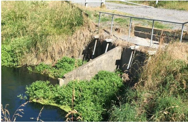
Figure 7.70. Two culverts with attached flood gates divide the upstream and downstream sub-sites along the Tutaekuri Waimate
