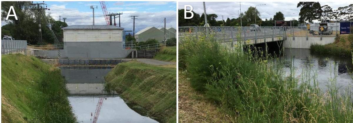
Figure 7.108. A: A pumping station divides the upstream and downstream sub-sites along Plantation Drain. B: A large box culvert beneath the Ford Road bridge lies 100m downstream of the pumping station.
