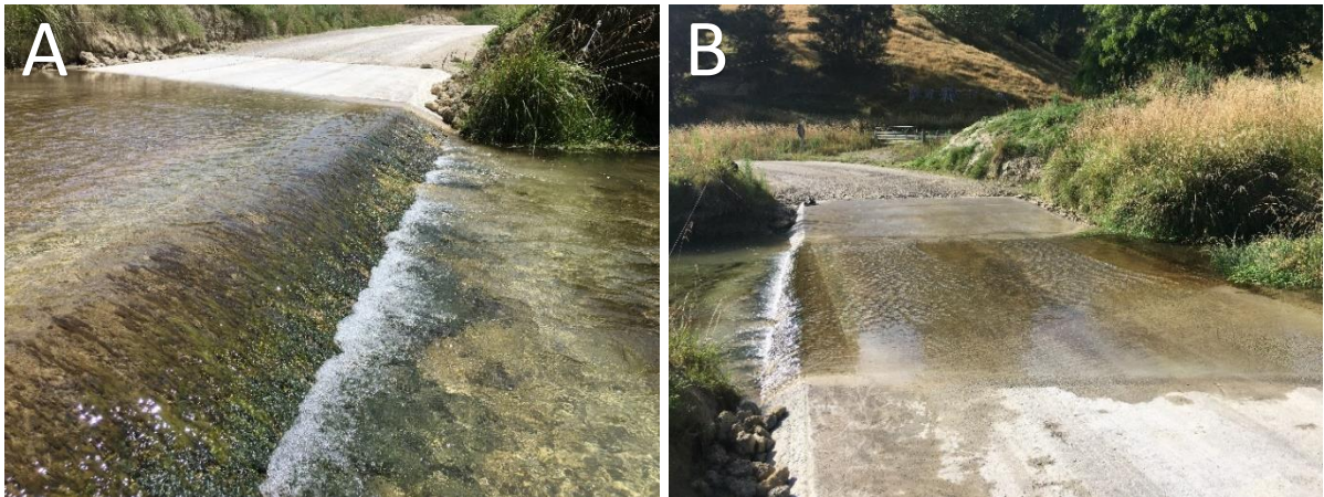
Figure 7.54. A ford divides the upstream and midstream sub-sites along the Pakuratahi Stream. A: The ford's drop causes may act as a potential barrier to upstream migrating fish. B: The ford crosses a dirt road which is used by heavy logging trucks.
