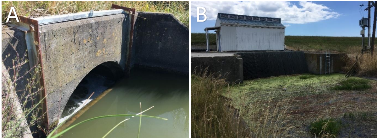
Figure 7.84. Two drainage structures lie along Muddy Creek. A: A Fish-Friendly Flood Gate (FFFG) divides the midstream and downstream sites. B: A pumping station divides the upstream and midstream sites.
