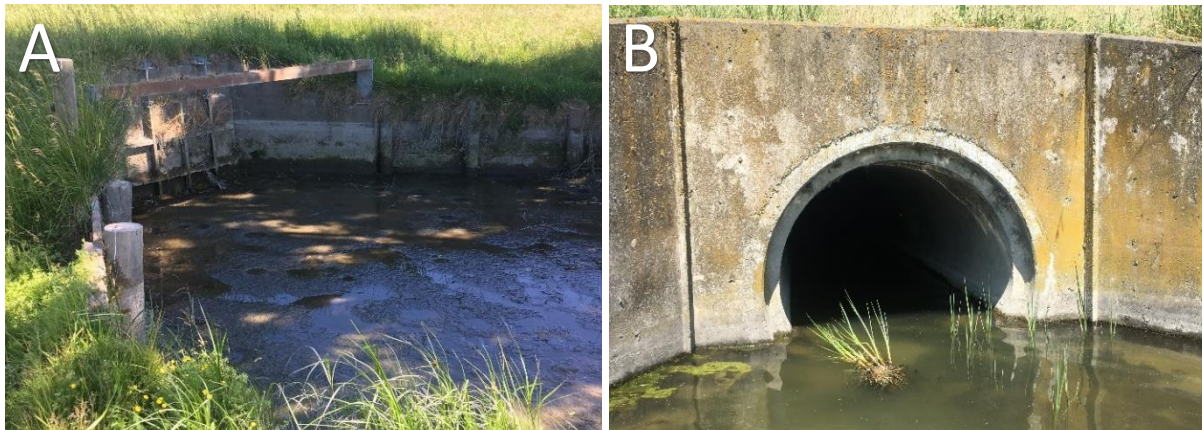
Figure 7.74. A flood gate and pipe culvert lie between the upstream and downstream sites along Pakowhai. A: The closed flood gate during a low tide. B: The inlet of the large pipe culvert, spanning ~2m in diameter.
