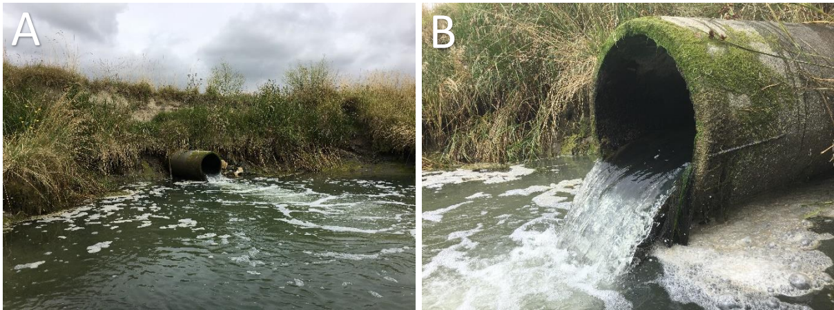
Figure 7.65. A pipe culvert divides the upstream and downstream sites along the Ngaruroro Backwash. A: The culvert's outlet is considerably smaller in size in comparison to the width of the downstream waterway. B: During periods of low tide, a drop forms beneath the culvert's outlet.
