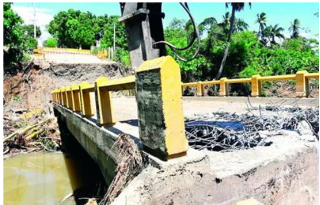
Fig. 2 Recent precast bridges collapse in the DR (Rodríguez and López 2007, Batista 2017)
