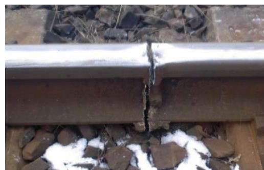
(b) Rail break caused by thermal contraction (Zwolski, 2012)
