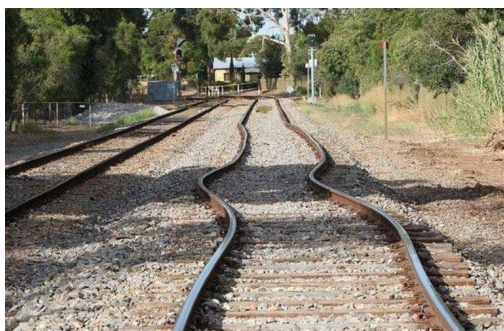
(a) Rail buckling caused by thermal expansion (Zwolski, 2012)
