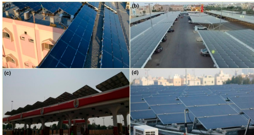
Figure 4. Solar projects in Kuwait: (a) Sawda bin Zamaa PV rooftop grid connected; (b) Al-Zahra Co-op Parking Shades PV Rooftop-Grid connected; (c) Al-Zahra Petrol Station PV Rooftop-Grid connected; (d) Azda bint alhareth School PV Rooftop-Grid connected. Adapted from [30].
