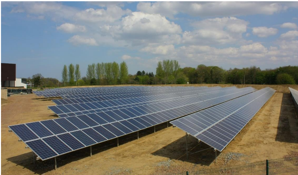
Figure 24 View from W of site (front of panels)
