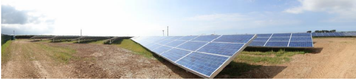
Figure 3 5MW Trenouth Solar PV Farm, Source: (Rugg, 2012)
