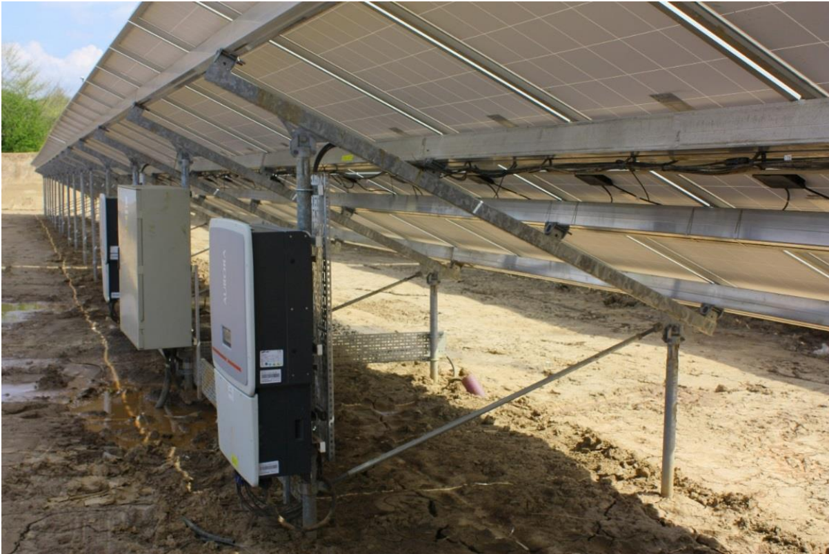
Figure 28 Inverter and AC Distribution Box Setup
