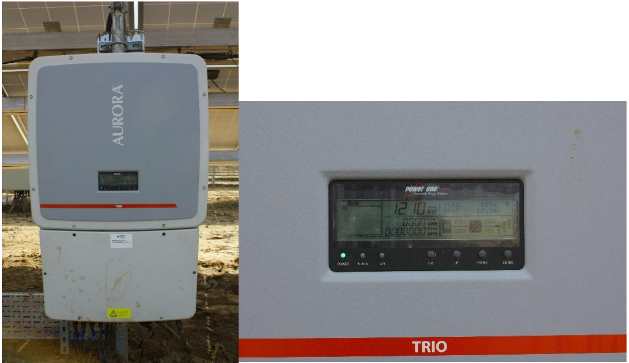
Figure 29 Front View of Inverter and Detail of Display Screen
