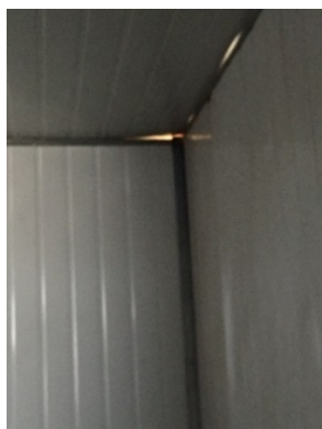
Fig. 5 Gaps between junctions [13]
