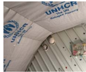
Fig. 17 Ventilation pipes closed [15]
