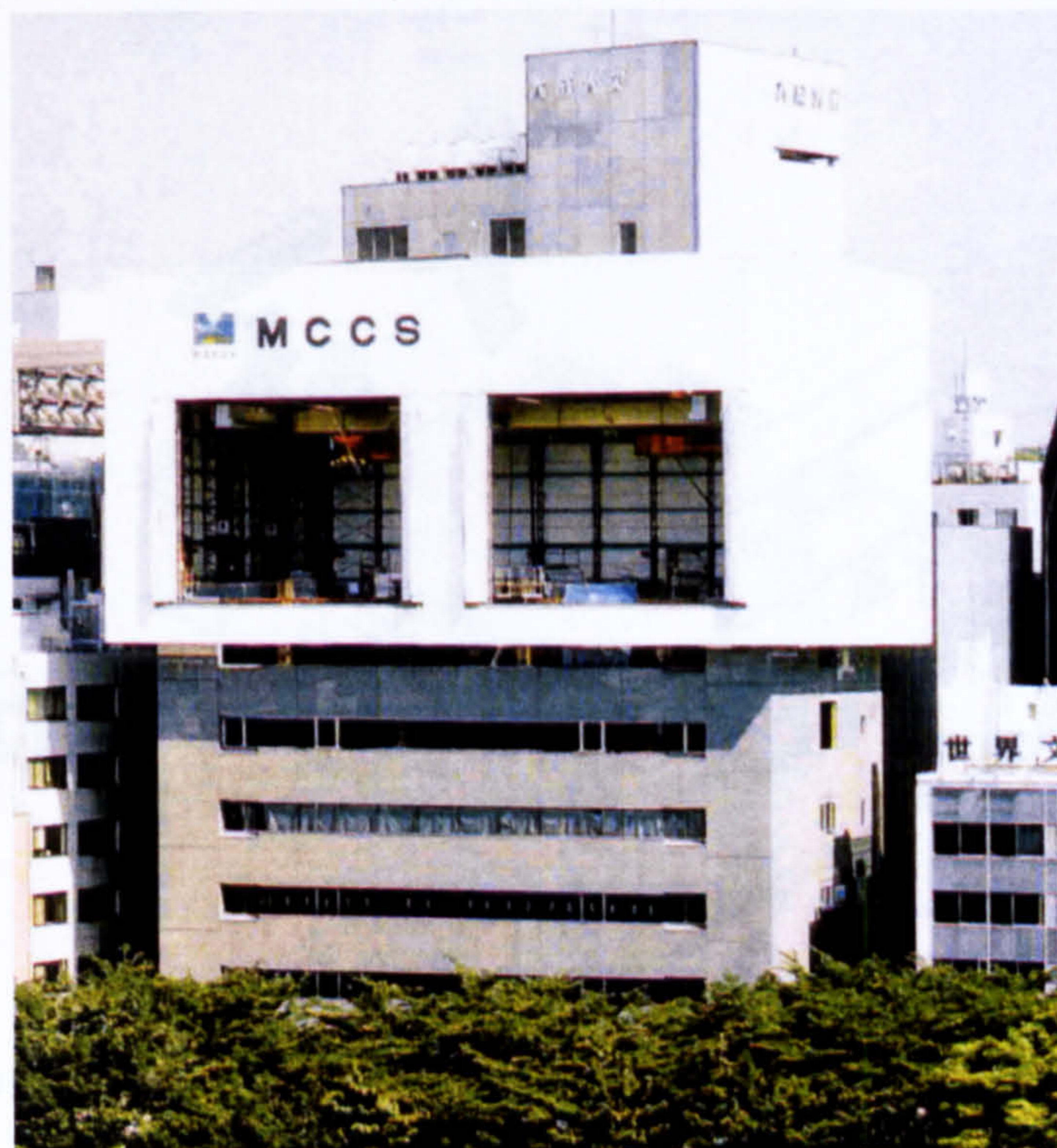
Figure 3.47: MCCS system exterior view Courtesy: Maeda Corporation
