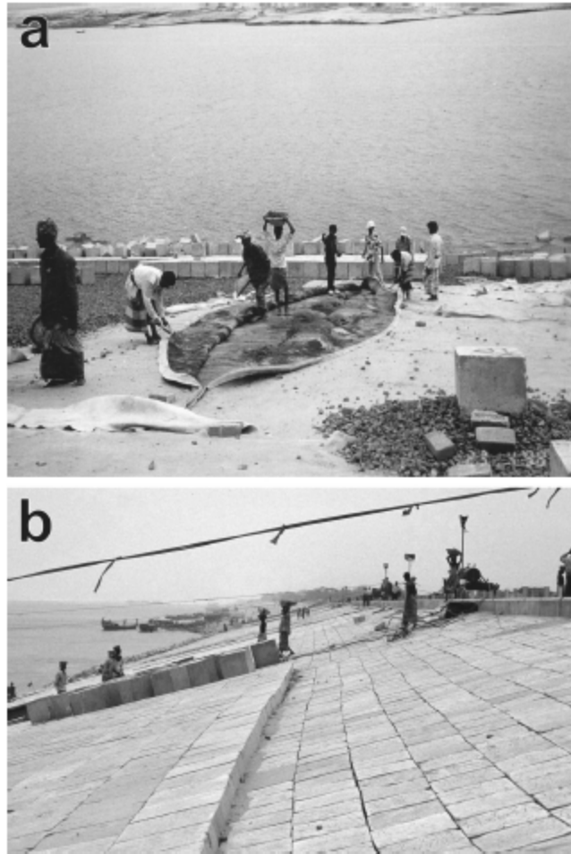
Figure 21.32 Construction of the B2 hardpoint at Sirajganj showing: (a) dredged river silt covered with geotextile membrane filter, then covered by broken brick and concrete cubes (photograph courtesy of Mr Bob Courtier, W.S. Atkins Ltd) and (b) 0.45 m 3 concrete blocks in place, view looking downstream from the hardpoint 'nose'
