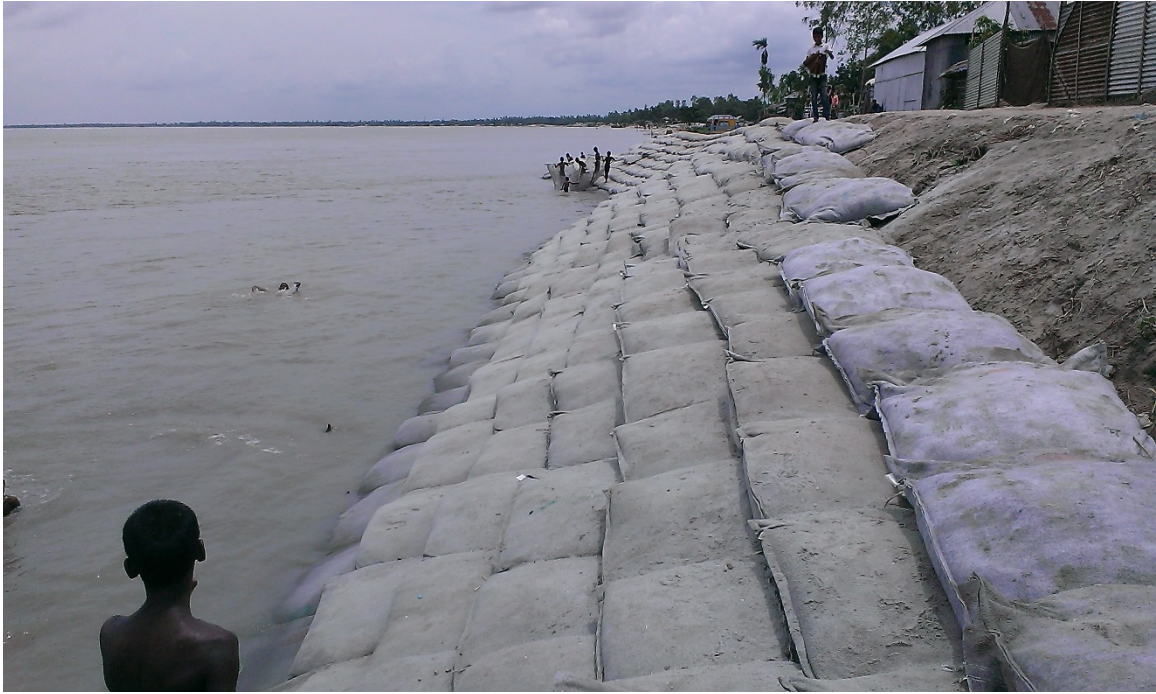
Figure 21.34. Sand-filled geotextile bags, or geobags, used for bank protection at Chauhali, Jamuna River. View looking upstream.
