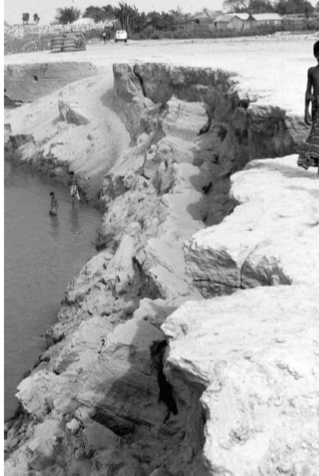
Figure 21.28 Large-scale slab failure by bank undercutting near Shailabari (~4 km upstream of Sirajganj). Photograph taken at low flow. During seasonal floods the water level would be up to bankfull.
