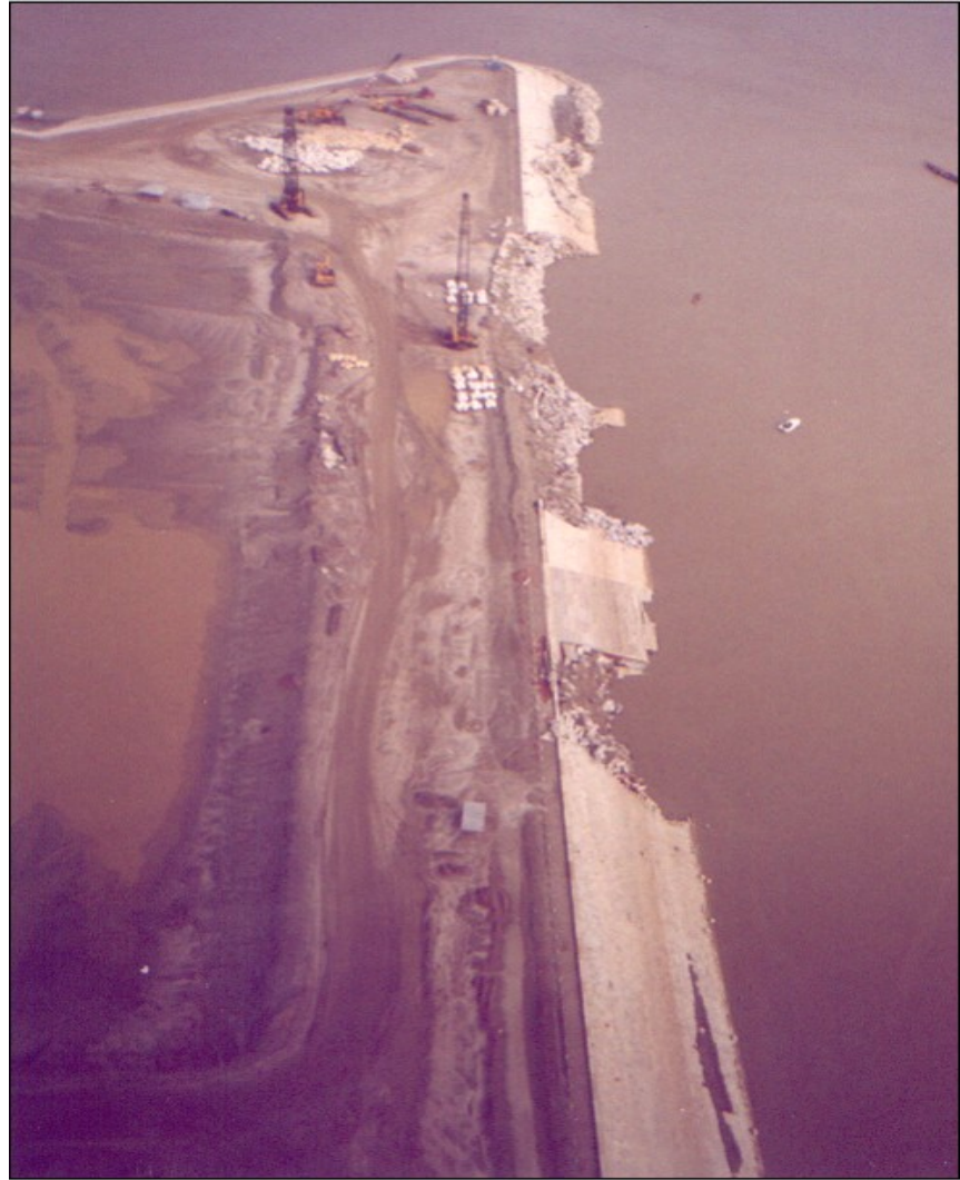
Figure 21.33. Image of the B2 hardpoint in 1998 showing the multiple failures formed at the height of the 1998 flood (photograph courtesy of Mr Bob Courtier, W.S. Atkins Ltd).
