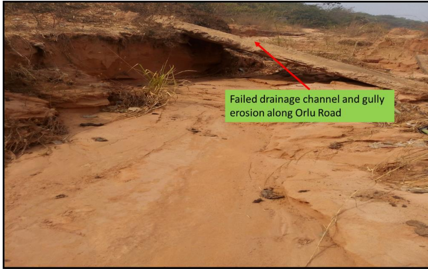
Figure A- 9-1 Failed drainage channel and gully erosion along Orlu Road, Owerri
