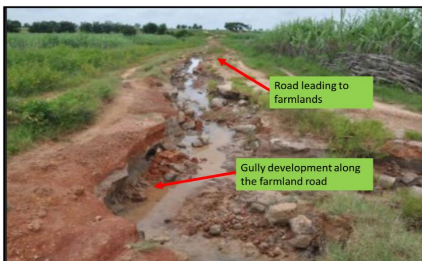
Figure 7-6 Gully development along road leading to farmlands in the watershed. Source: Author's fieldwork: 05 42' 05''N 007 02' 35.8''E
