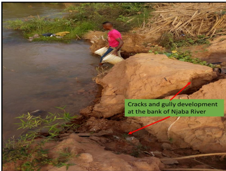
Figure A-9-8 Cracks and gully development along the foot path of Njaba Riverbank Source: Author's fieldwork
