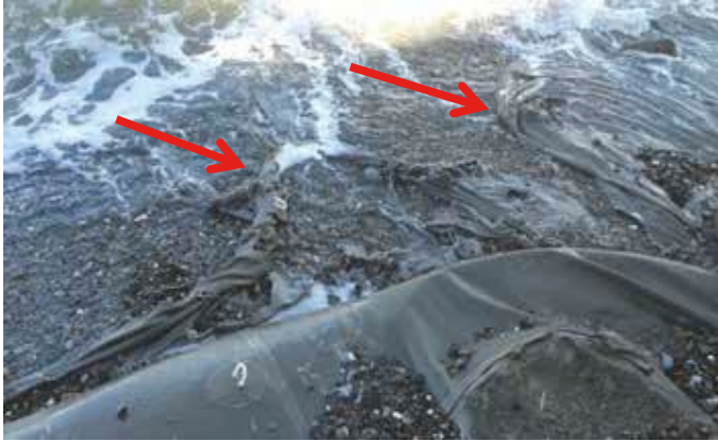
Figure 8 - Some sacks of geotextile cloth containing sand were completely destroyed (red arrows) by sea storms.
