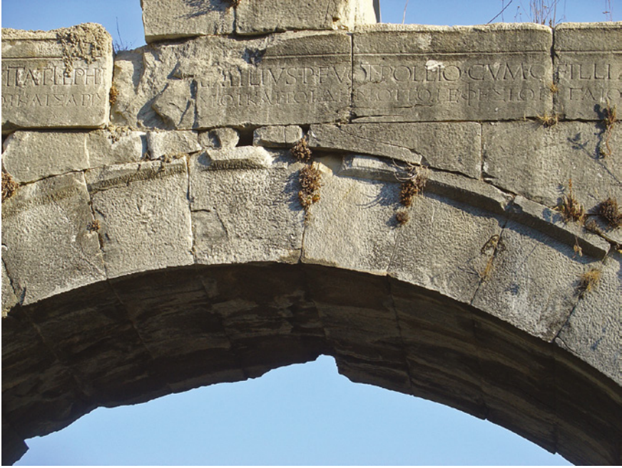
FIGURE 8.3 Detail with inscription (IK Ephesos 12, 402) of a section of the Aqua Throessitica, Ephesos
