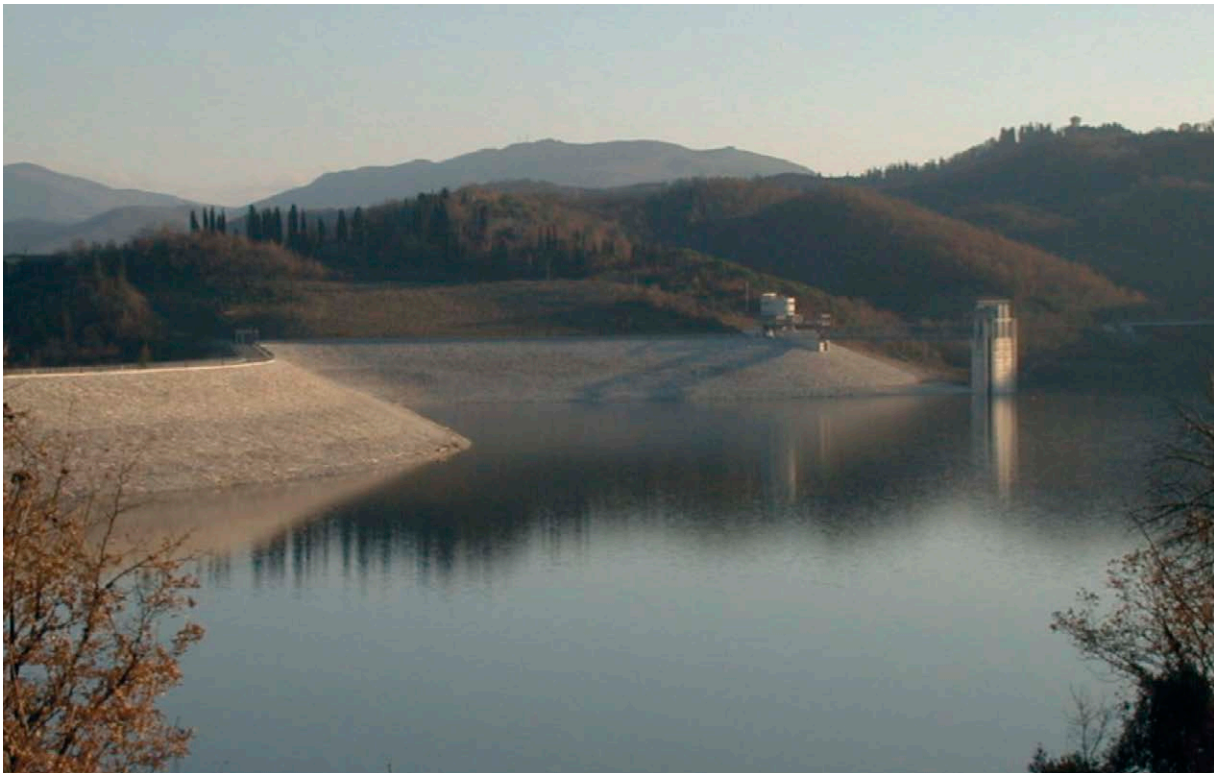
Fig. 3-11. The Bilancino earthfill dam in the upper Sieve basin (Photo reproduced from Caporali et al., 2005).
