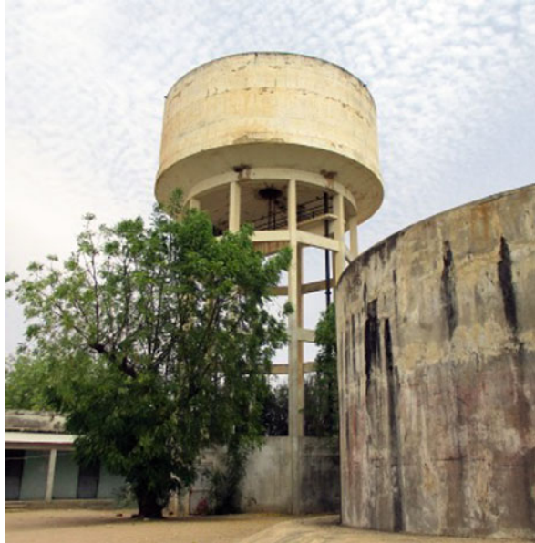
Fig. 4.2 Typical water tower maintained by ASUFORs in rural Senegal. (Photo by Ikemi)
