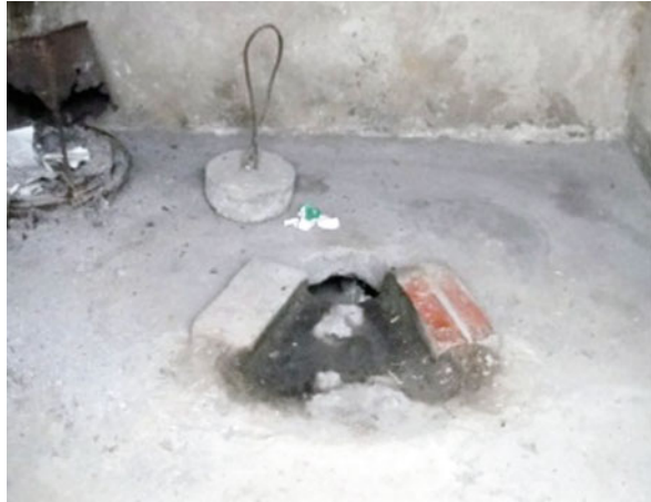
Fig. 8.7 A dry toilet storing excreta in a fecal chamber under the floor slab. (Photo adapted from Harada and Fujii (2020))
