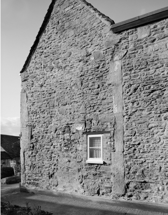
FIGURE 21.3 View of the east wall of the former chapel of St Helen at Malmesbury in 1992 © CROWN COPYRIGHT. HISTORIC ENGLAND ARCHIVE (REF. BB/15936).
