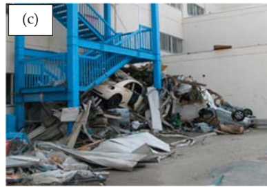
Figure 3. Damage from cars: (a) a dump truck collided against a warehouse at the Kirinda fishing port in Sri Lanka, (b) a passenger car collided against a shop at Miyako in Japan, and (c) many cars were pushed against the corner of a school building at Sendai in Japan.
