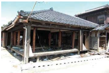
Figure 26. Wooden house, inundation depth 2 m, wall destruction, Kitaibaraki City.
