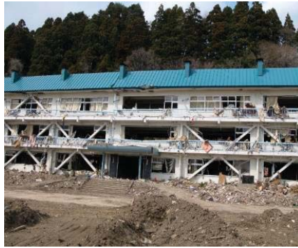
Figure 24. Reinforced concrete building, inundation depth 8.5 m, Rikuzentakata City.
