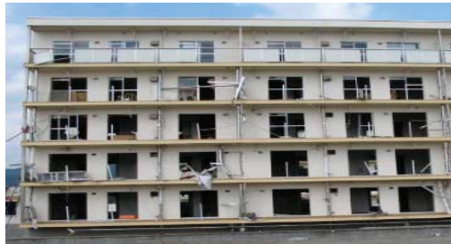
Figure 22. Reinforced concrete building, inundation depth 10 m, Rikuzentakata City.
