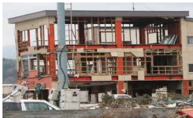
Figure 23. Steel building, inundation depth 7.5 m, panel wall destruction, Yamada-cho.
