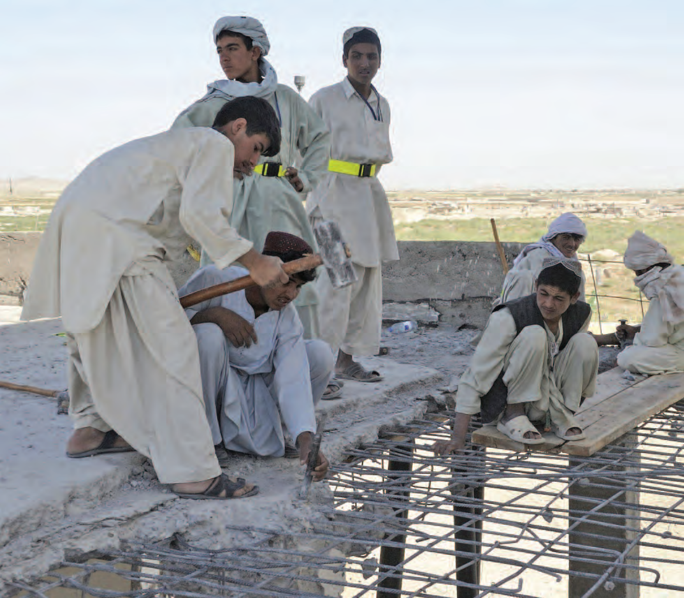
Residents of Deh-e-Bagh work on the renovation of the Dand District Centre. (Photo by Cpl Jonathan Barrette)
