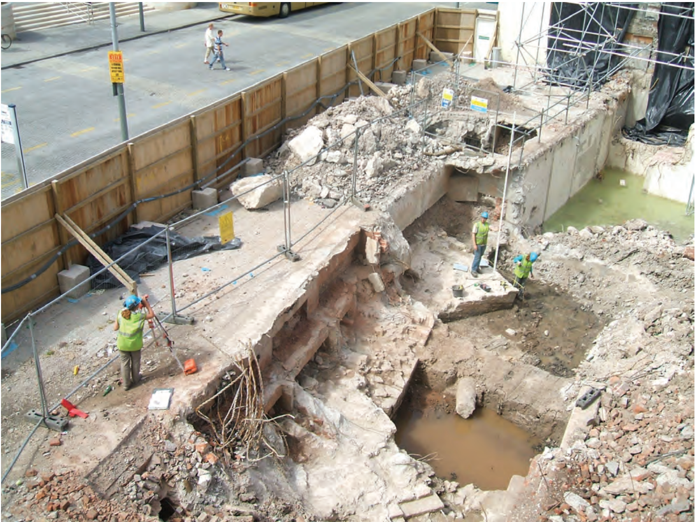
Figure 6.36 Part of the Marsh Wall adjacent to Broad Quay as exposed in 2006
