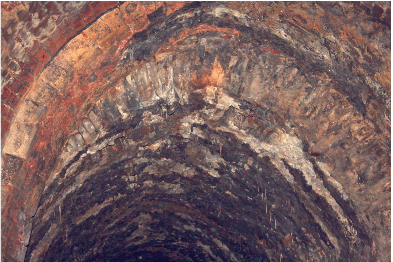
Figure 6.26 Underside of the bridge spanning the moat under Castle Street (photograph Nigel Baker)
