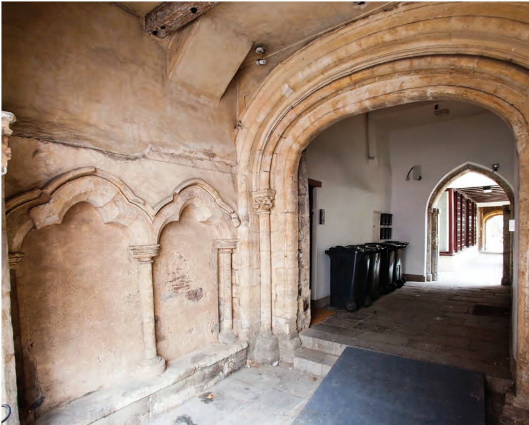
Figure 5.31 St Bartholomew's Hospital: south doorway to 12th-century hall and 13th-century arcade (photograph D Martyn)
