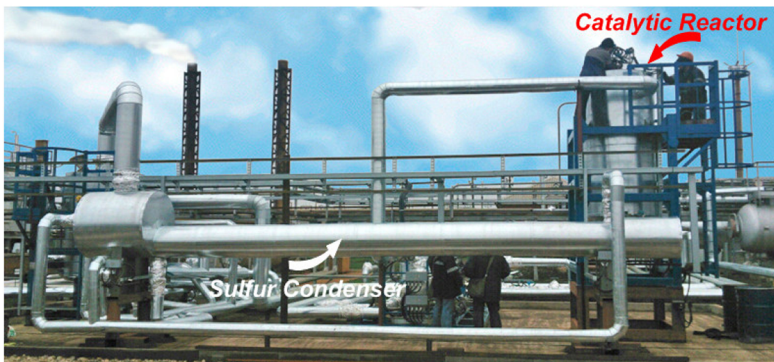
Figure 29. Industrial APG purification plant by direct catalytic oxidation.
