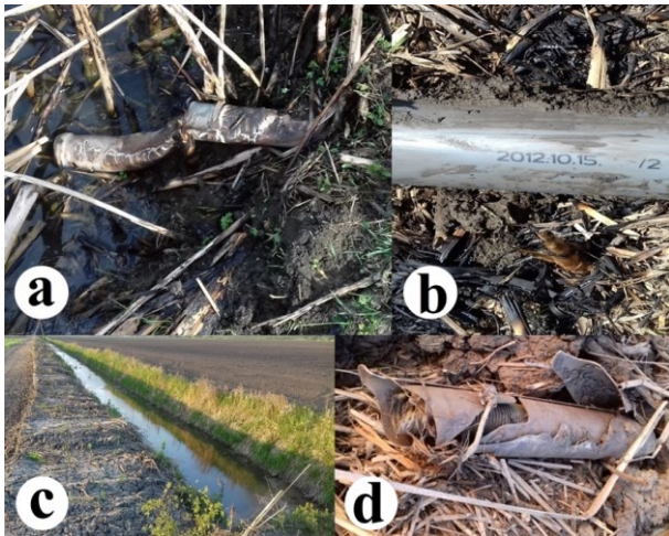
Fig. 7 Typical conditions of the drain pipes at the Mezőtúr study site: (a) melted PVC drain outlet in the channel side slope, (b) a few years old relocated drain pipe outlet, (c) open channel after sludge removal in Csanytelek, (d) ruptured drain pipe in spreaded sludge
