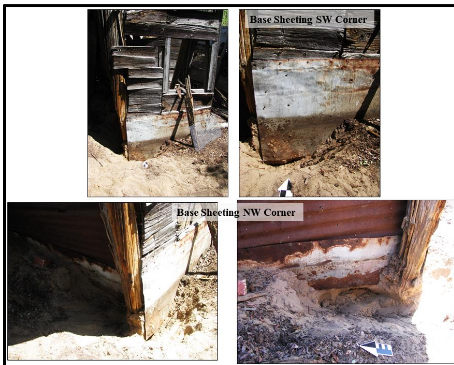
Figure 24. Upper left-south and west side (with window). Upper right-southwest corner photo showing partially buried tin sheeting on lower base of the coop wall, and lower left and right- alternate views of the upper and lower (buried) tin sheeting at the building's northwest corner.
