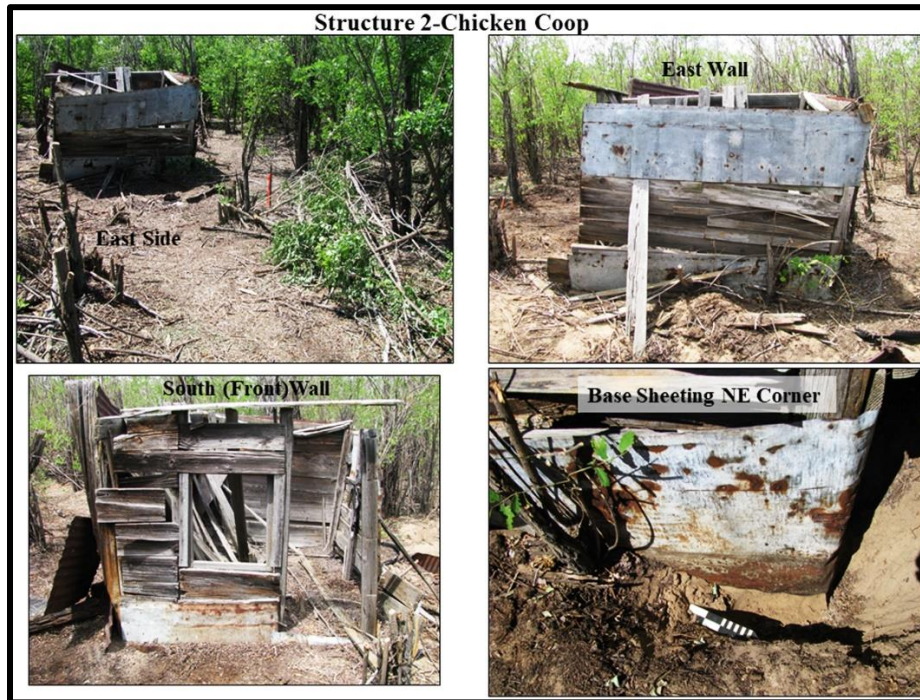
Figure 23. Alternate east and south views of the Squire Brockman chicken coop with a close-up of the tin sheathing extending from the east wall plank base below the ground surface.
