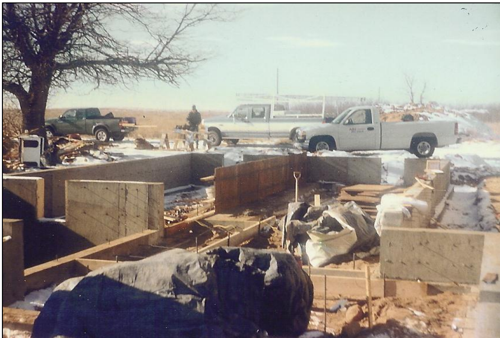
Figure 22. View of the new foundations of the Jackson House in 2001. Photo courtesy of Kevin Murray, Bellvue, Colorado.
