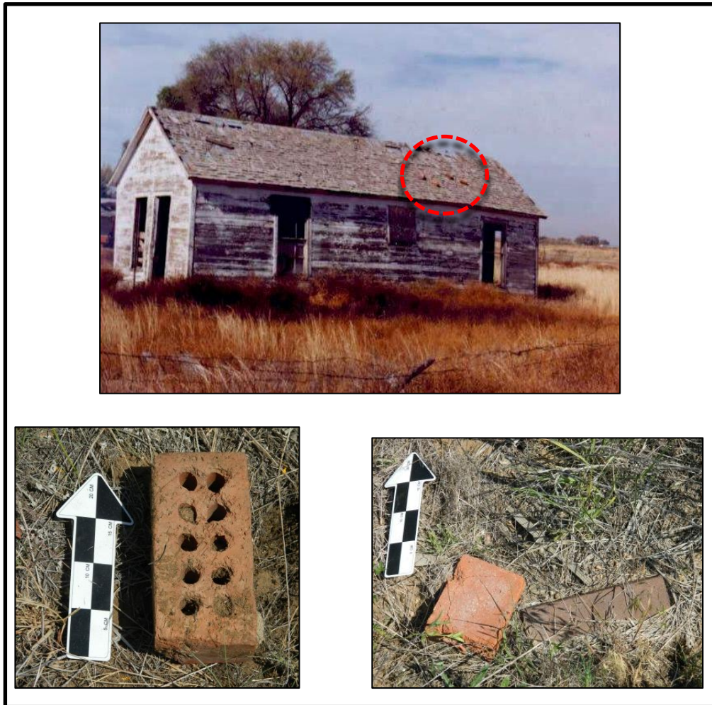
Figure 9. 1994 OAHP site form photograph showing the Block 4 House from the south east east with red bricks on the roof from earlier chimney demolition and salvage. Two 2011 photos at the bottom of the figure show bricks found at the north end of the house footprint.
