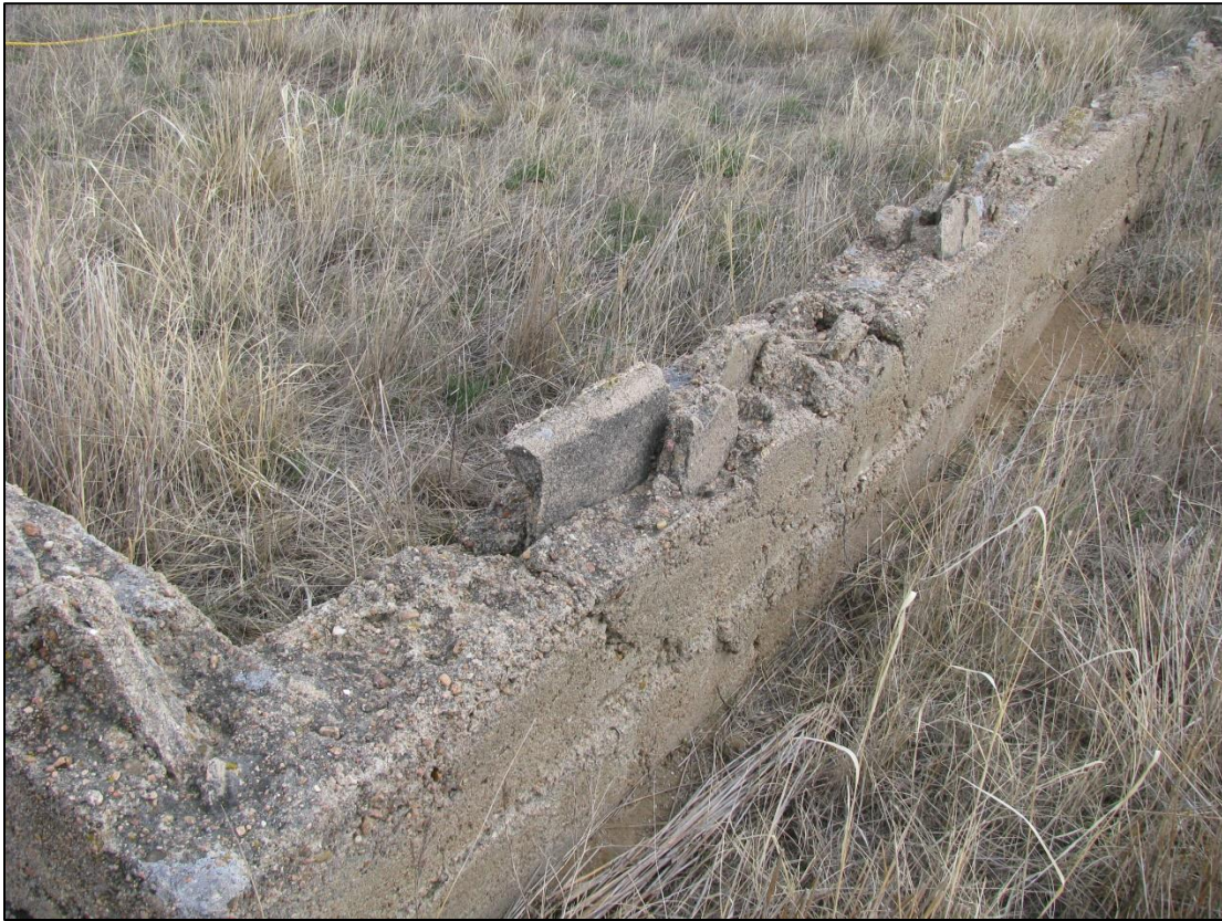
Figure 15. Section of the concrete wall showing broken slabs and chunks of broken concrete set into the formerly wet concrete along the top of the wall, creating an uneven jagged effect incompatible with supporting a building floor and walls.
