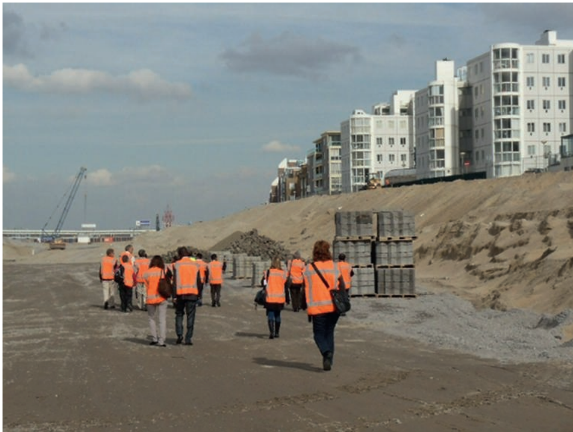
Case Study 9.7 Figure 1 Multipurpose dike in Scheveningen, a coastal resort near the Hague, the Netherlands.
