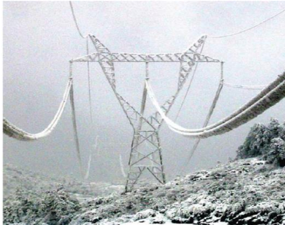
Figure 56: Ice accumulation on an HV transmission line [159]
