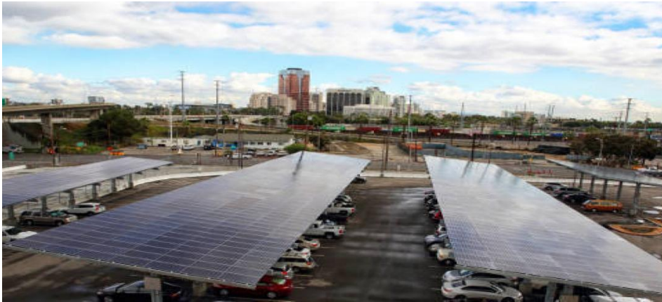
Figure 10: Solar panels on carport of Long Beach (“Mitsubishi Electric”, 2016).
