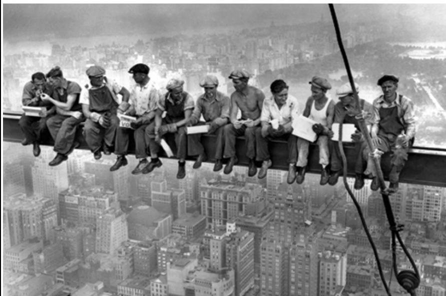
Ironworkers eating lunch on a beam of a skyscraper under construction. Rockefeller Center Construction, New York, NY (1932). 95
