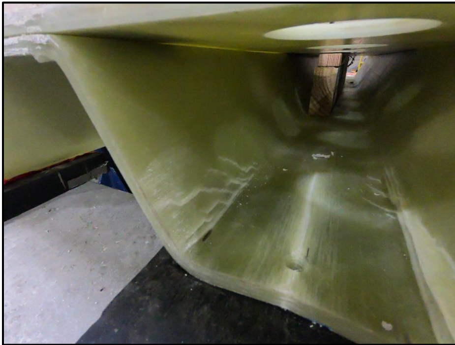
Figure 91: Inside of Corrugation at Support of Failed Panel 1
