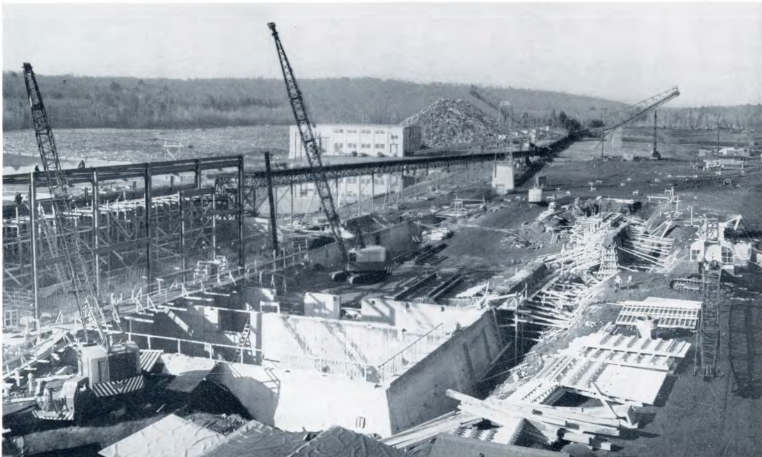
Construction activity at the East Millinocket Mill: foundations for the new grinder room.
