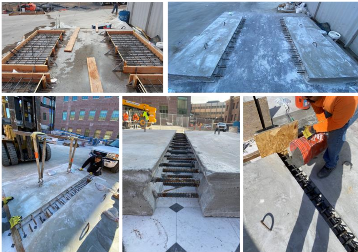
Figure 6-5 Photographs from the fabrication process and illustration of the sequence of constructing test specimens.
