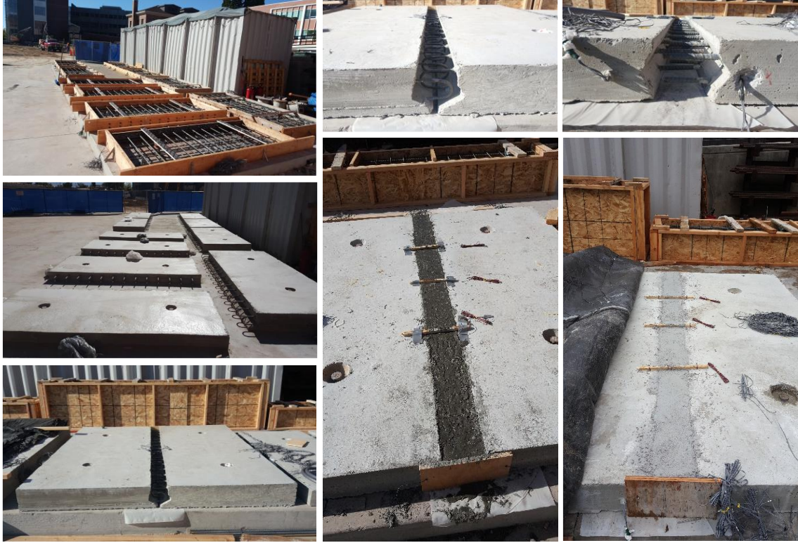
Figure 2-7 Photographs that illustrate the various construction stages and sequence of precast deck assemblies with UHPC and PC field joints
