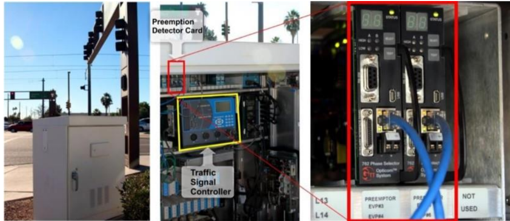
Figure 4 Preemption Detection Card in the Cabinet
