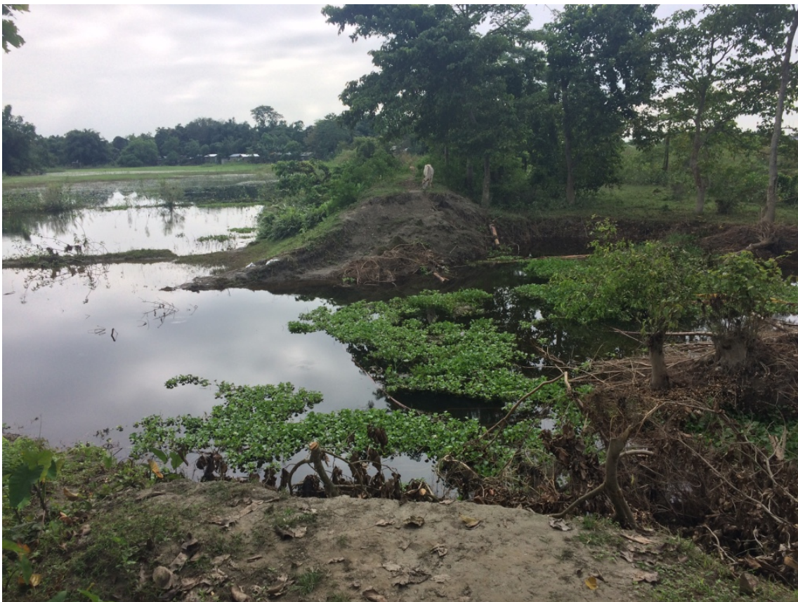
Fig. 2.3. Breached embankment two weeks after the event, with flood water receded (source: author).
