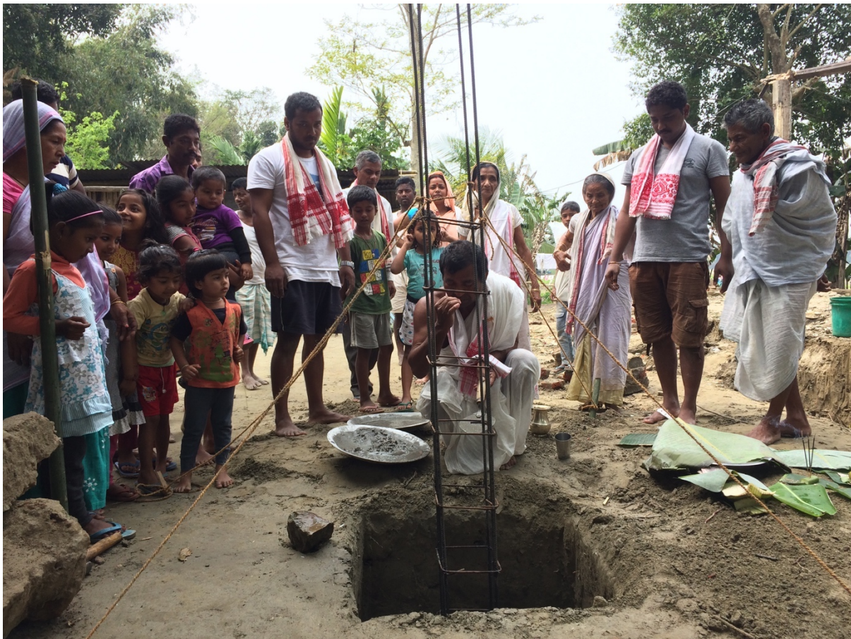
Figure 3.2. Centre ground, a Deori or officer of the village namghor (prayer hall), or one who distributes prasad , ceremoniously pours the first trowel of cement into the base of what will become a reinforced concrete post on the auspicious front eastern side, which is also the direction of prayer. The deori (otherwise referred to as biloniya ) had just led the family and close kin and neighbours in a naam (sung prayer) before blessing ( ahirbaad ) the start of construction.
