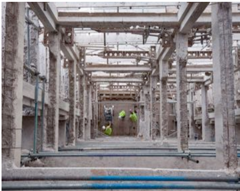
Figure 30: Exposed reinforcement during the period of the renovation. Courtesy of Urban Splash.
