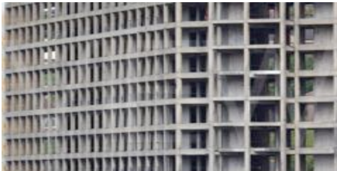
Figure 45: The bare structural frame of concrete was revealed during the reconstruction. Image courtesy of Urban Splash
