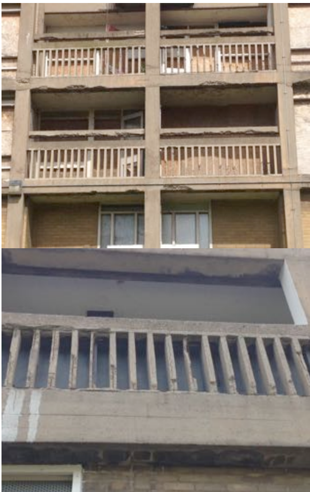
Figure 17 a and b: Spalling on the balustrades and the horizontal structural beams. Image author's own.
