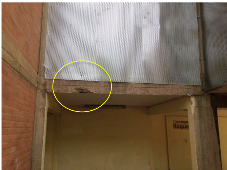
Figure 28: Spalling on a structural elements, revealing the rebar underneath. Image author's own.
