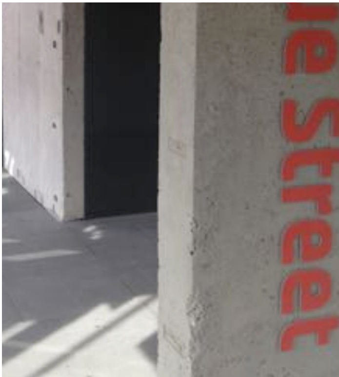
Figure 29: The edges on the columns after they have been repaired.. Image author's own.
