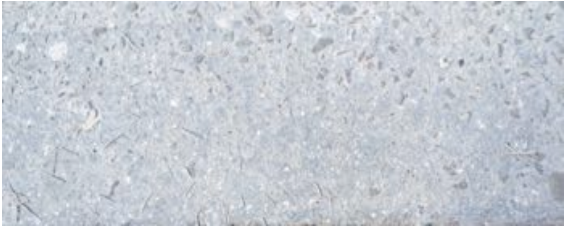
Figure 1: Concrete on the Manchester Metrolink with fibre reinforcement coming out of its surface. Image author's own.
