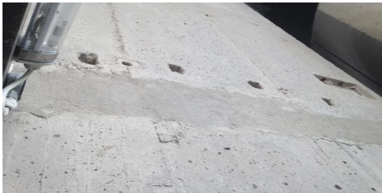
Figure 52: Dents and marks on the concrete of Park Hill in places where the concrete has been rehabilitated. Image author's own
