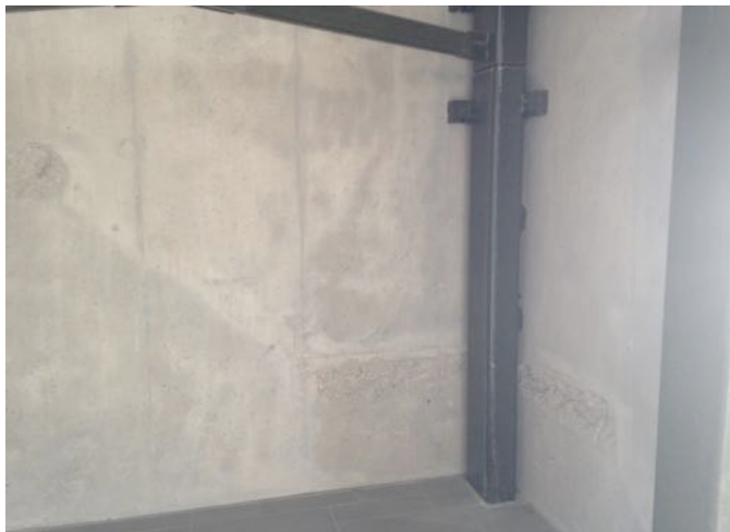
Figure 55: Visual inconsistencies resulting from elements that have been removed. Image author’s own
