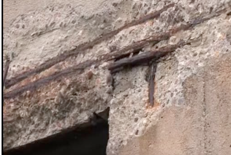
Figure 41: Spalling on a column to beam connection before rehabilitation. Image author's own
