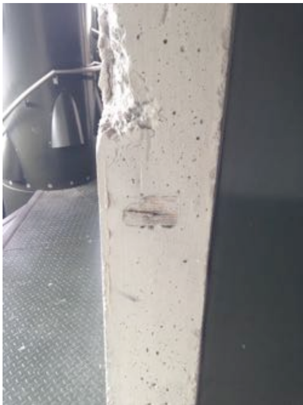
Figure 18 Spalling on a column at "street in the sky" level Image author's own.
