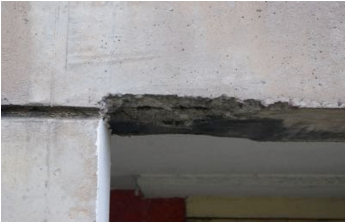
Figure 22: Spalling on the edge of a beam in Park Hill
