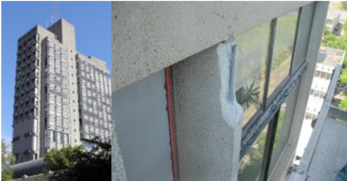
Figure 25: Peabody Terrace and the spalling concrete louvres on the building. Image by Brunner/Cott, taken from metropolismag.com (Moss, 2012)
