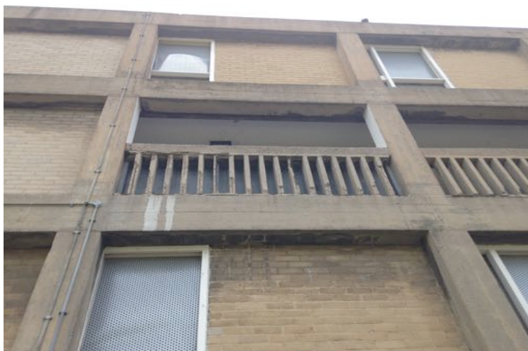
Figure 27: The original balustrades in Park Hill were too wide to comply with current regulations. Image author's own.
