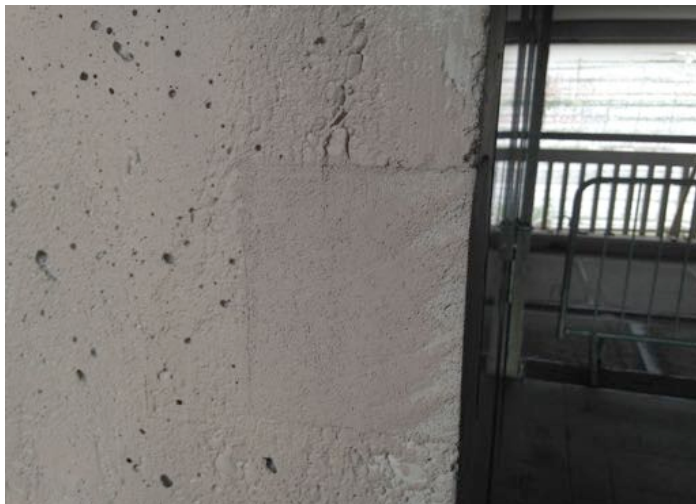
Figure 51: The repaired concrete in Park Hill is clearly visible: where there has been a repair, a neatly cut square area of the material has been removed and has been replaced by a fresh material, different in texture. Image author’s own.
