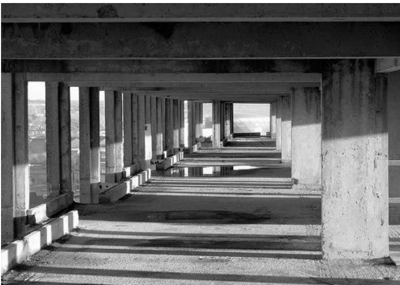
Figure 39: Park Hill stripped bare to the structural frame. Image courtesy of Urban Splash.
