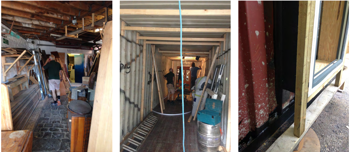
Figure 6.1.2 - L to R, Strip the Willow , using waste wood as framing internally and externally.
