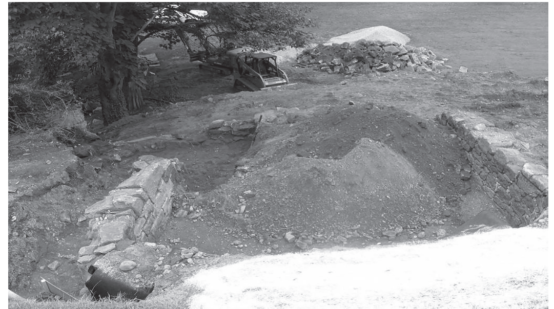
Figure 7. Overview of the Sentry Box Icehouse site after mechanical exploration, looking east towards the river. (Photo by Dovetail Cultural Resource Group, 2008.)
