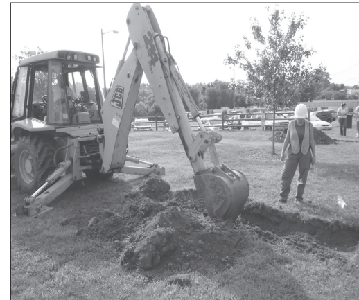
Figure 4. Excavating a backhoe trench at the Fredericksburg Riverfront Park; trench location based on archival data. (Photo by Dovetail Cultural Resource Group, 2013.)
