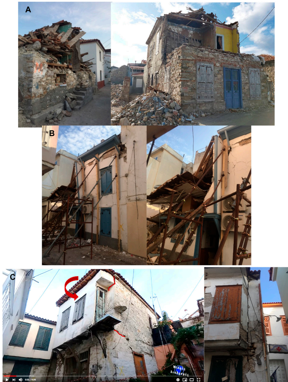
FIGURE 3 | Examples of damage to timber framing in timber-masonry structures. (A and B) : progressive failure of the upper floor timber framing and the roof [DG4-DG5]; (C) Overturning of the jetty in timber-masonry structures [picture on the left from Mikres Diadromes Samou, 2020] [DG3] (all in Samos, Greece).
