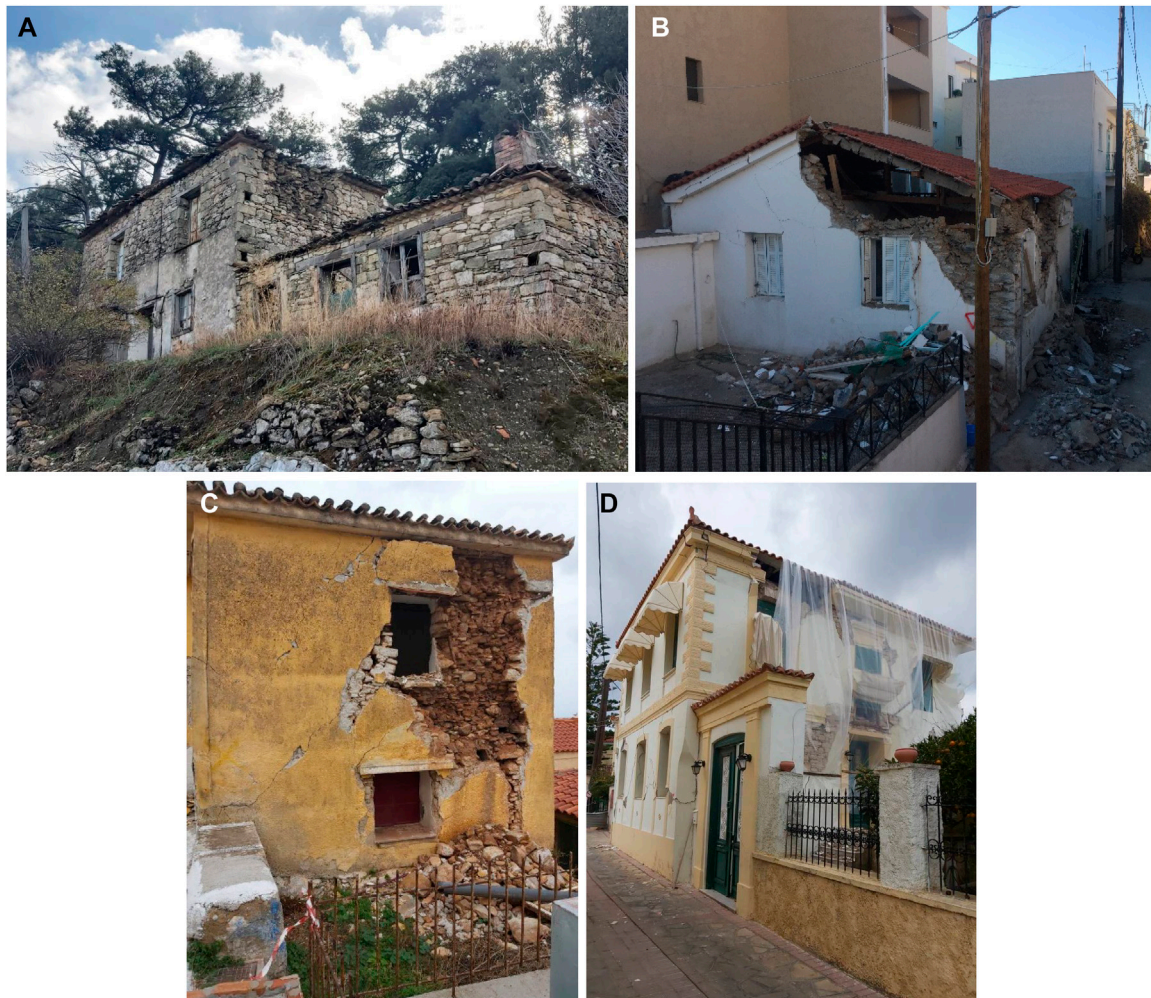
FIGURE 5 | Examples of out-of-plane failure in masonry structures: (A) Partial overturning of the external leaf; (B) Corner failure and partial overturning of gable; (C) : Out-of-plane failure of the external leaf of a multi-leaf masonry wall with mud mortar; (D) Out-of-plane failure of a brick wall [DG3-DG5](all in Samos, Greece).
