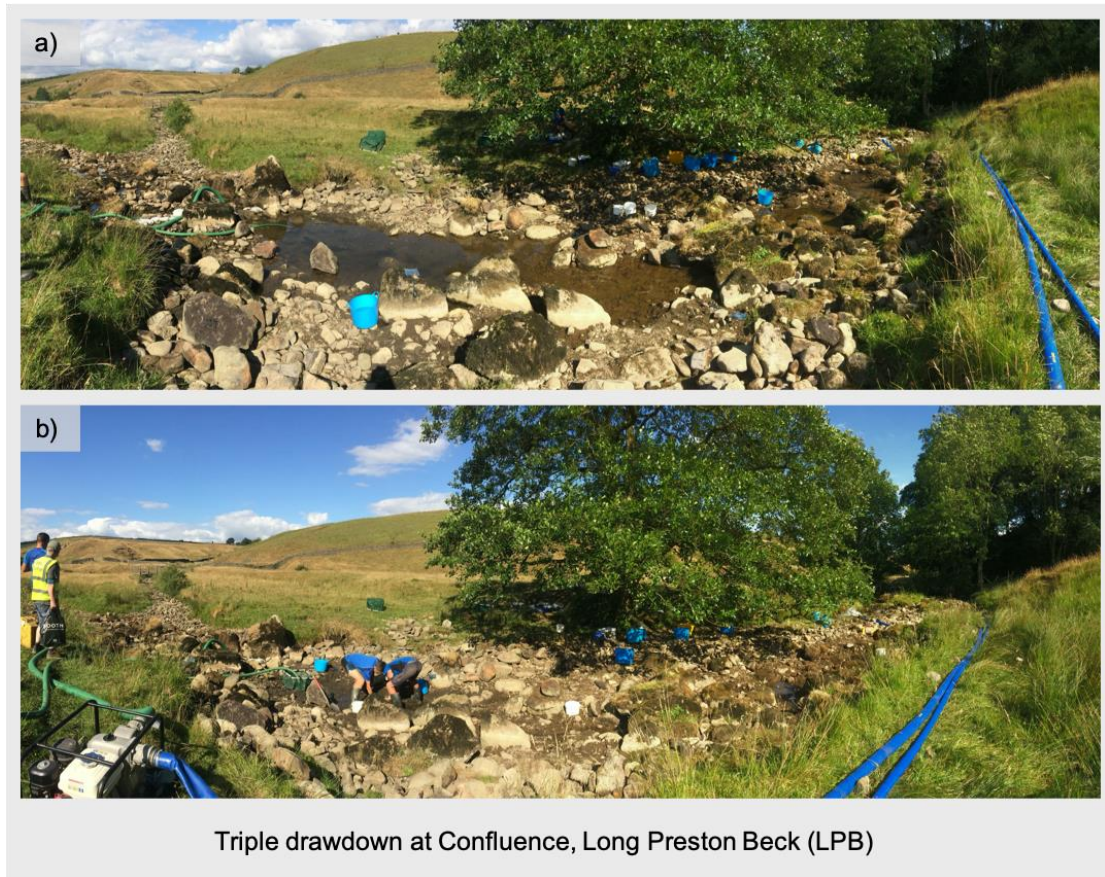
Figure 2.12 Triple Drawdown (TDD) at Confluence, Long Preston Beck (LPB), a) before dewatering and b) during dewatering.
