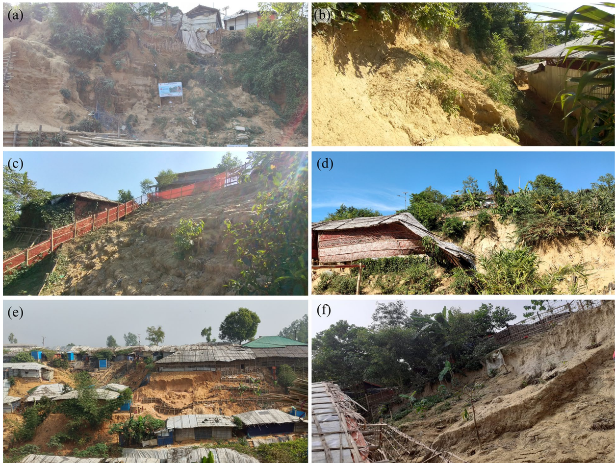
Fig. 3 Landslides in the Kutupalong Rohingya Camp (photos taken during the fieldwork). a Camp 18 (slump). b Camp 4 (rotational slide). c Camp 20 (creep with polygonal tension cracks). d Camp 17 (slump/debris flow). e Camp 8E (slump). f Camp 5 (rotational slide)
