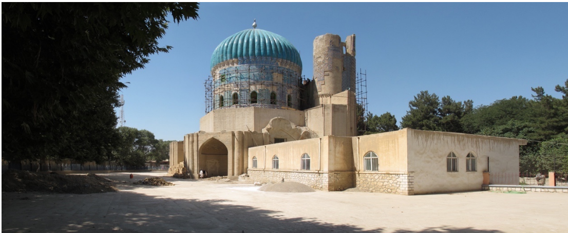
FIGURE 16 THE KHWAJA PARSA SHRINE, BALKH, SHOWING THE ADJACENT MOSQUE ON THE SOUTH WING, 2012. PHOTOGRAPH COURTESY THE AGA KHAN TRUST FOR CULTURE
