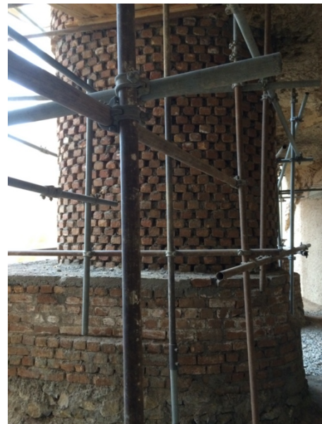
FIGURE 9 CONCRETE AND BRICK SUPPORTS FOR THE PROTECTIVE PLATFORM FOR THE NICHE OF THE EASTERN BUDDHA, BAMYAN, JUNE 2015. PHOTOGRAPH C. WYNDHAM
