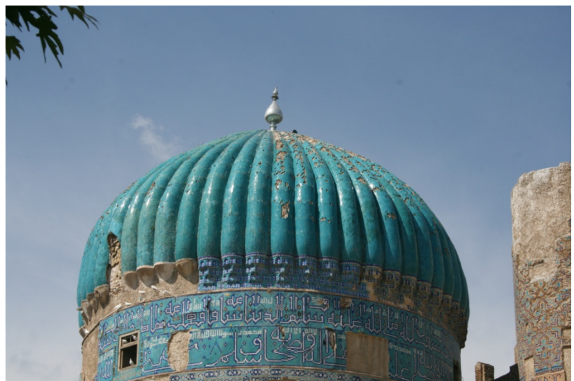
FIGURE 20 THE TIMURID-ERA DOME OF KHWAJA PARSA SHOWING THE LOSS OF TILES. PHOTOGRAPH COURTESY THE AGA KHAN TRUST FOR CULTURE
