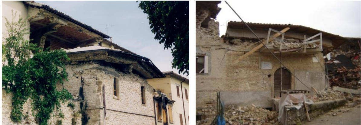
Figure 2-3 Failure due to excessive weight of RC roof structure built on poor quality masonry walls (credits to Maddaloni 2016).
