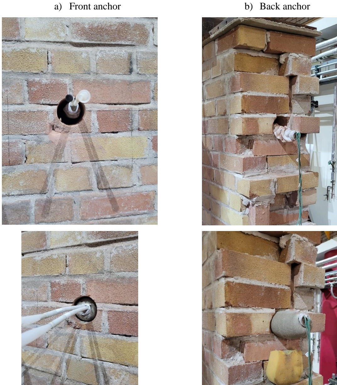
Figure 5-31 Installation of D-GAS and grout injection a) front anchor b) back anchor
