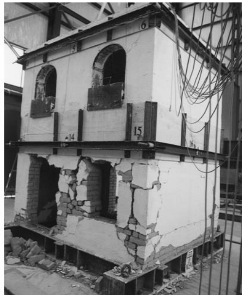
Figure 2-2. Shear failure of masonry structure reinforced by means of concrete bands (Benedetti, Carydis, and Pezzoli 1998)
