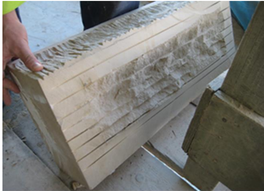
Figure 2.7: Example of poor practice; overzealous removal of replacements stone to enable fixing
