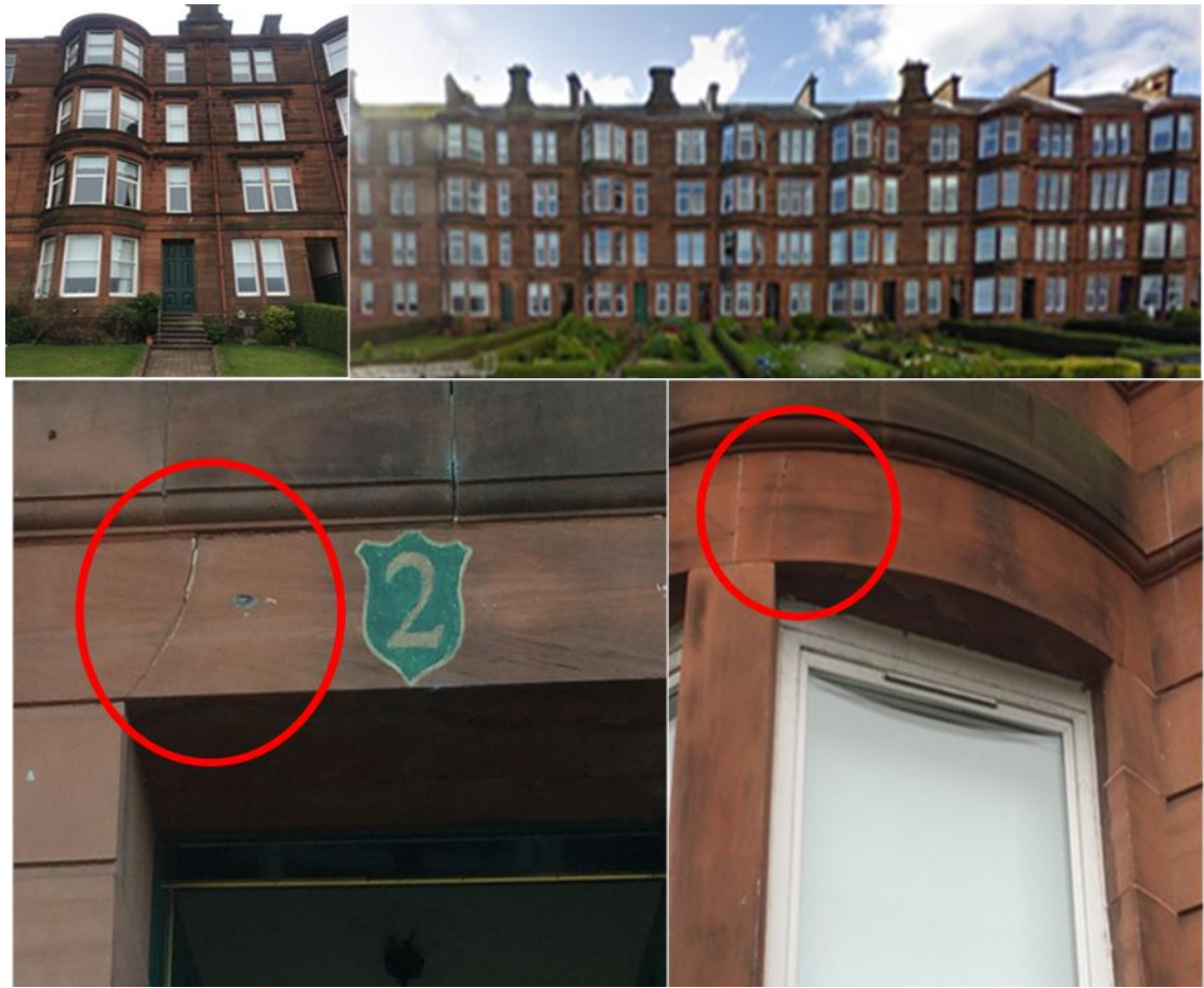
Figure 8.2: Top left: Project “A”: Front Façade; Top right: Pre-1919 Block of Tenement Flats; Bottom left and right; Examples of Loss of Structural Integrity
