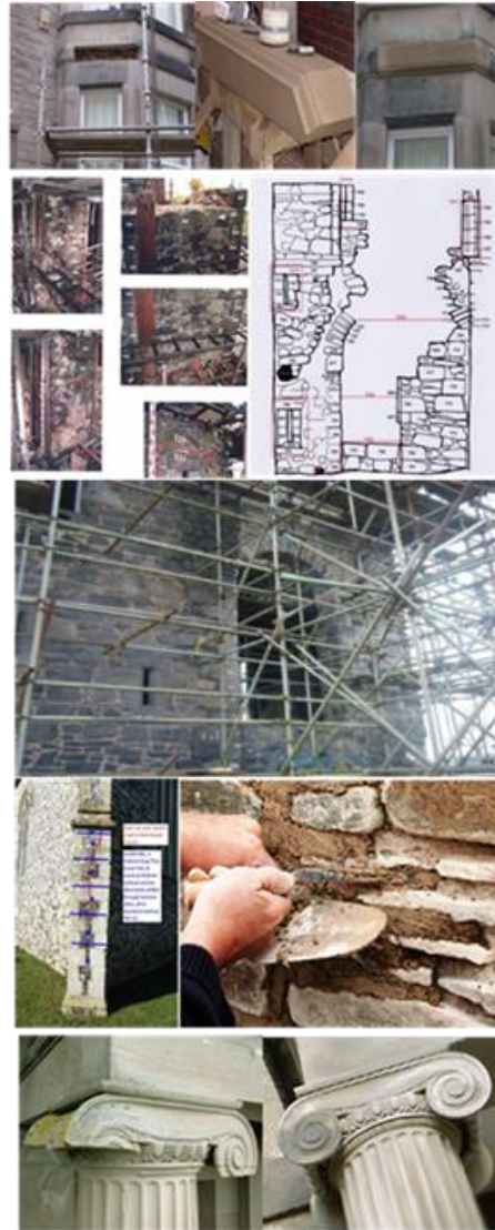
Figure 2.2: (i) full stone replacement; (ii) dismantling, record and re-build (iii) pinning and consolidation, (iv) mortar replacement, and (v) “plastic” repair
